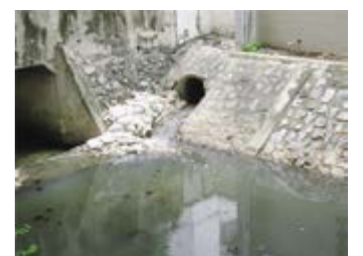
Treated wastewater directly discharged from a condominium into an urban canal
